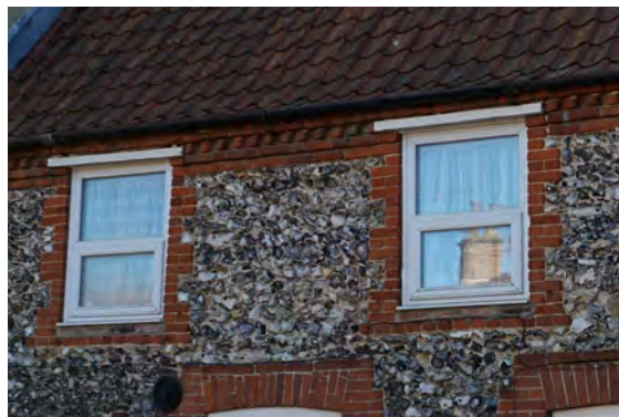
Inappropriate uPVC windows
