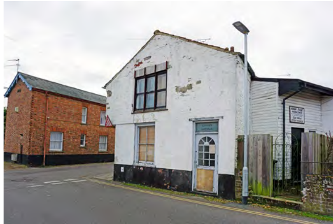
Building in poor condition on Cley Road
