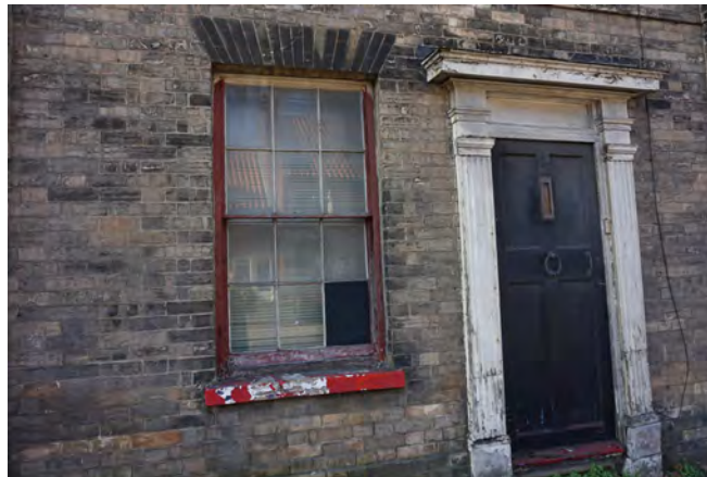
Timberwork in poor condition
