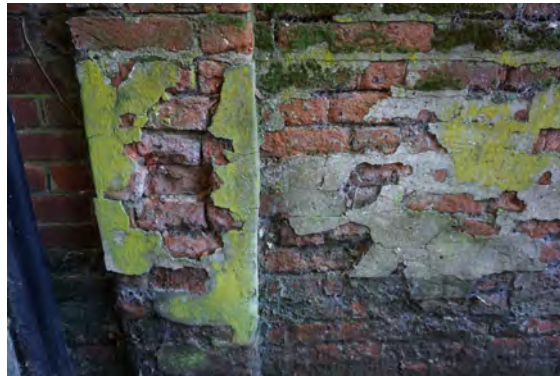
Inappropriate cement repairs causing further deterioration to the brickwork behind
