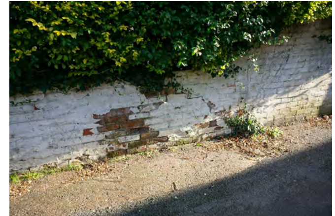
Flaking paintwork, cracking and vegetation growth to a wall
