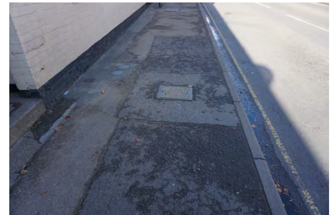
Patched tarmac pavement
