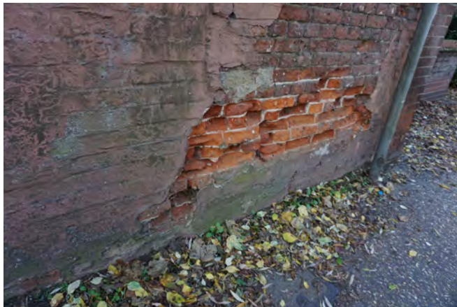
Brickwork worn from water backsplash from adjacent road
