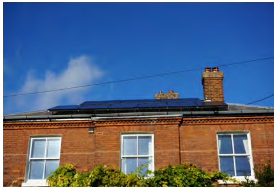
Solar panels on a roof facing the street
