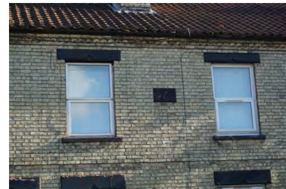
Inappropriate uPVC windows
