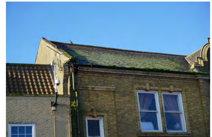
Vegetation growth in gutters
