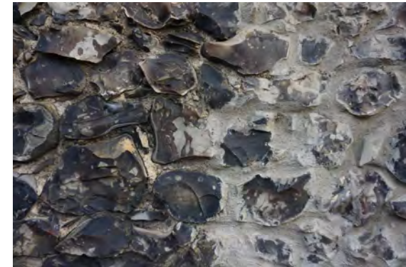
Poor cement repairs to flintwork on the right, with original lime mortar on the left
