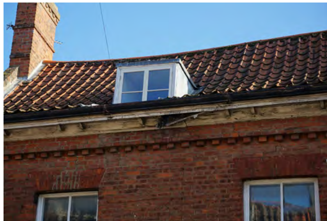
Decaying timber cornice
