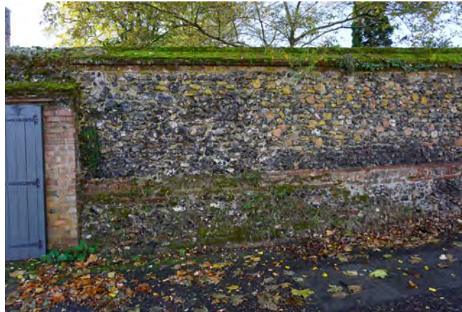
Wall with vegetation growth and inappropriate cement repairs
