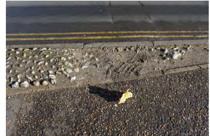
Missing cobbles on Lynn Street
