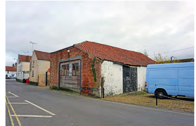
Building in poor condition on Cley Road
