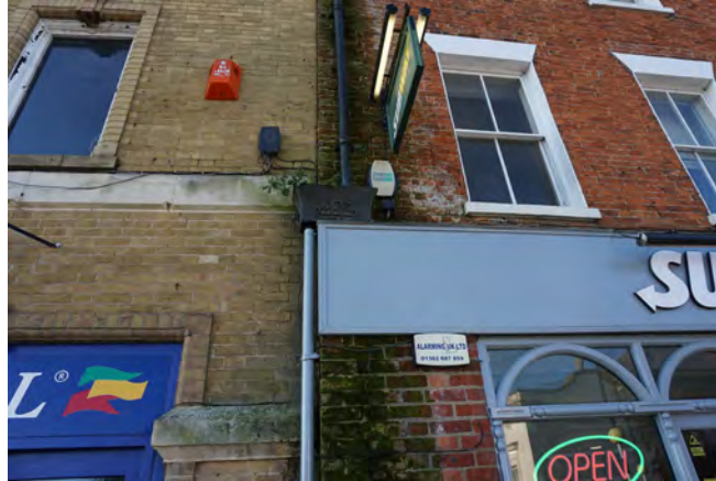
Water ingress and moss/vegetation growth due to blocked gutters and hoppers
