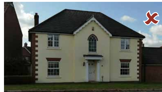
Poorly proportioned house with central projecting gable, regular floor to floor heights and a concrete tiled roof that appears heavy. Windows are side and top hung casements with no reveals. Render contrasts crudely with red brick lintels at ground floor only and quoins.
