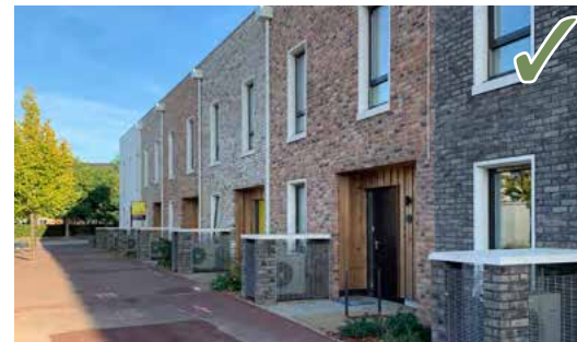
Air Source Heat Pumps are positioned at the front of dwellings to enable easy servicing, but are enclosed to screen them and avoid dominance when viewed from the street.
