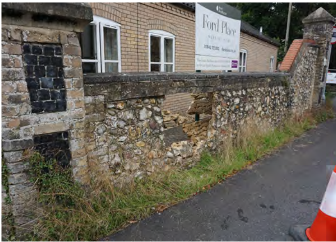
Flint wall in poor repair outside Ford Place
