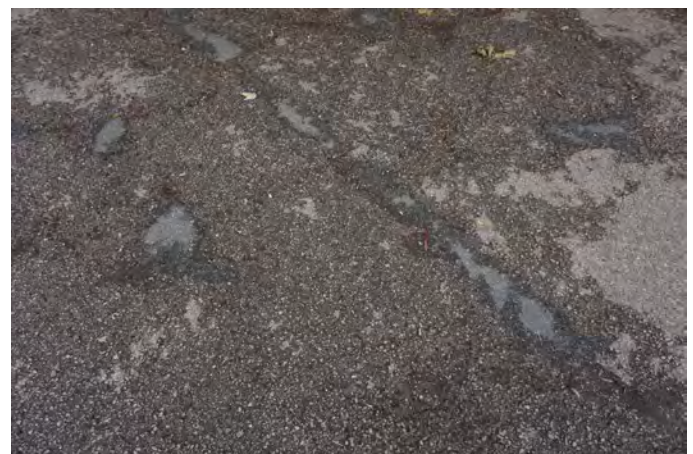
Cracked and uneven surface by the Old Mill
