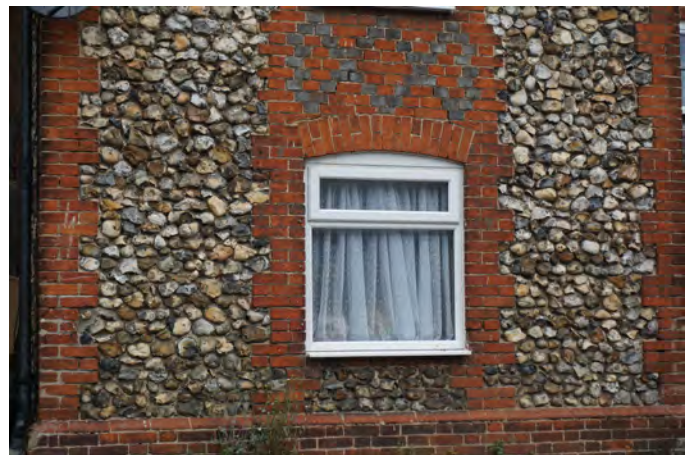
Inappropriate uPVC window
