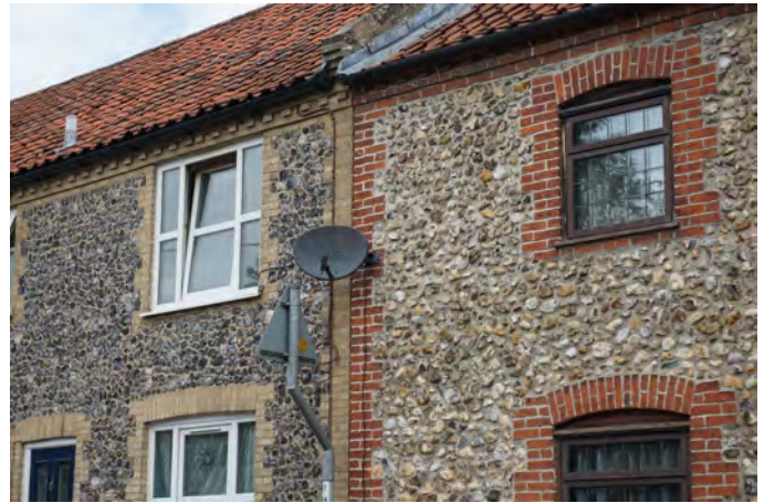
Inappropriate uPVC windows
