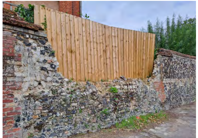
Wall in poor repair with fence inserted in opening on Star Lane
