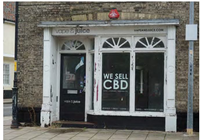
Flaking paintwork on timber shopfront in the Market Place
