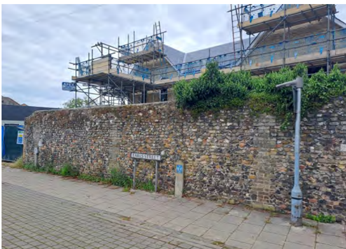
Vegetation growing on wall on Earls Street, with some evidence of it having been removed.
