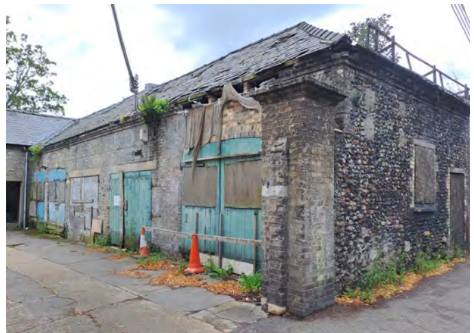
29a Bury Road with loose slates, vegetation growing within, missing brickwork and boarded up windows and doors
