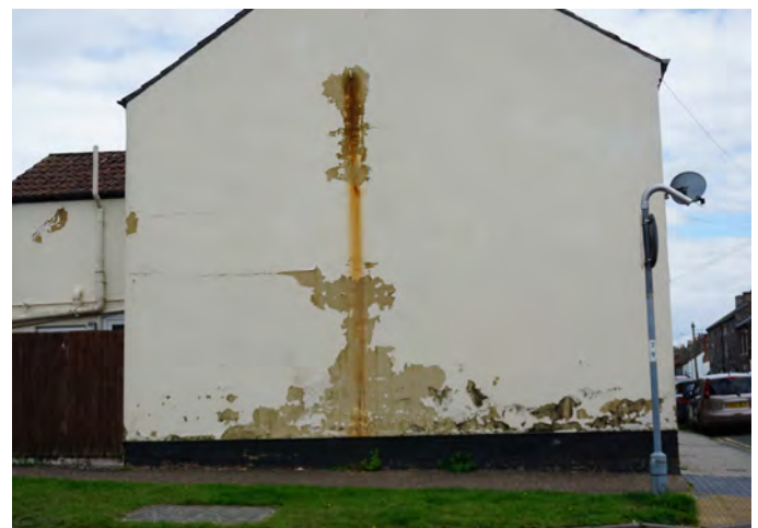
Flaking paint on 17 Castle Street
