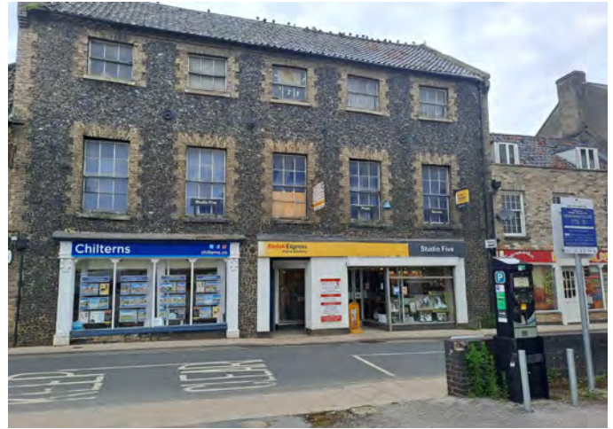
12-16 Bridge Street with rotten and blocked in sash windows giving the building a vacant appearance on the upper floors
