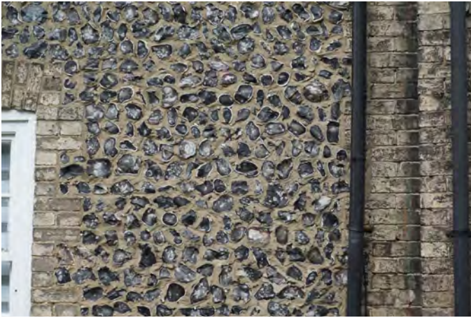
Inappropriate cement render on houses on Magdalen Street
