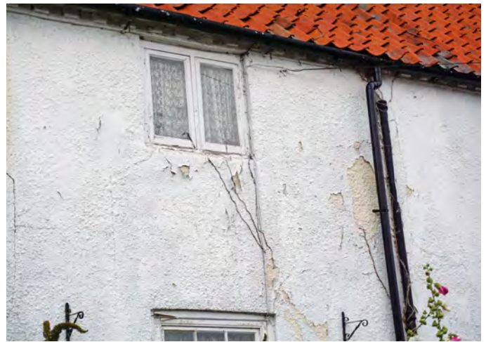
House front in poor condition on Magdalen Street
