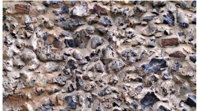
Inappropriate cement repointing of flint
