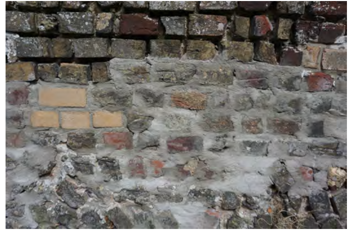
Poor repairs to brickwork including the insertion of inappropriate bricks
