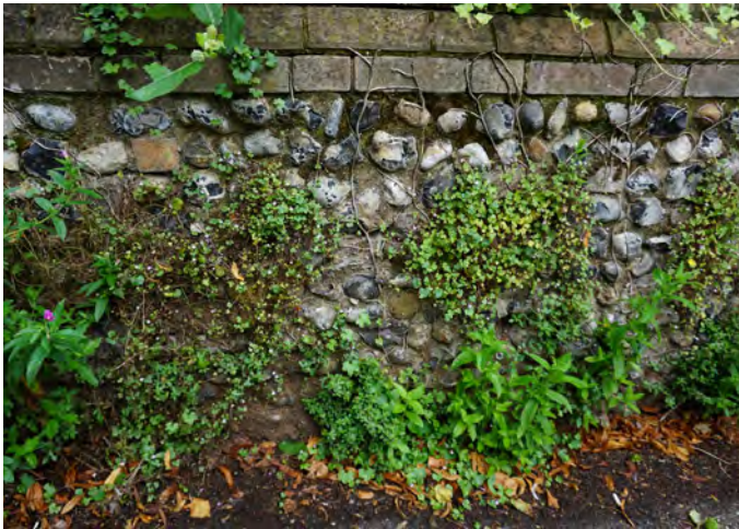
Vegetation growing on wall opposite the Old Mill
