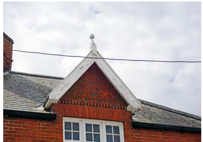
Flaking paintwork on the bargeboards of a building on Old Market Street
