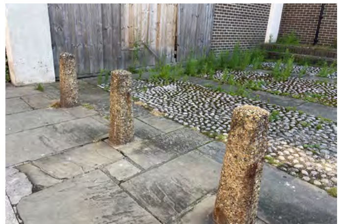
A combination of poorly maintained surfacing by the Bell Inn on Bridge Street
