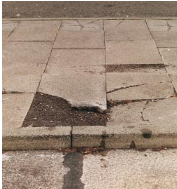
Damaged footways are a major source of injury. Courtesy: The Pedestrians Association.
